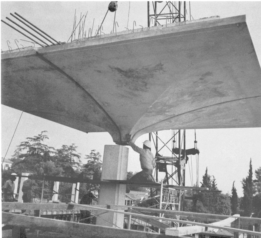
FIRST UMBRELLA —Huge crane very carefully lowers first Dining Hall umbrella into position while brave man directs its descent.
